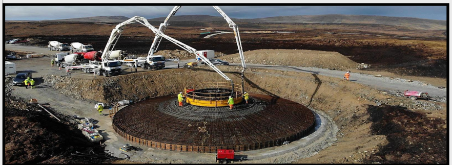
Above: The concrete & steel base of a Turbine. These structures are the same as are being proposed in all the Bute Energy Cambrian Mountains Wind Farms.
